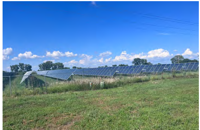
Community solar farm located in southeast Lexington.
