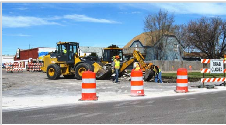
Workers begin to remove concrete at N 5th & Jackson. N 5th from Jackson to Grant will be replaced, as will Grant from N 5th to Hwy 30.
