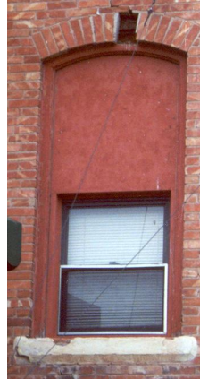
Example of an inappropriate window replacement
