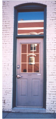
Example of an inappropriate commercial replacement door.
