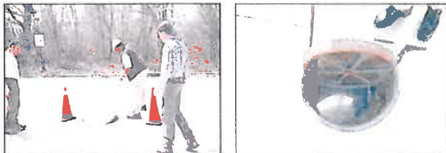
Figure 55: Manhole observation (left) indicates a sewage discharge. Source is identified at an adjacent sewer manhole that overflowed into the storm drain system (right).
