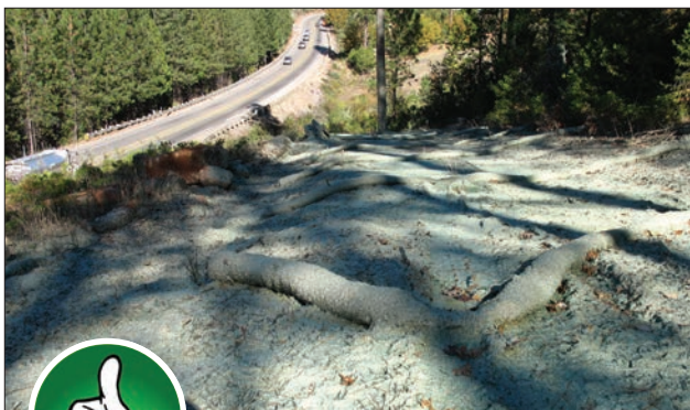
Fig. 4-9. Hydroseeding of large slopes is always more effective when done in combination with sediment control measures such as the fiber rolls shown here. Source: RBF Consulting
