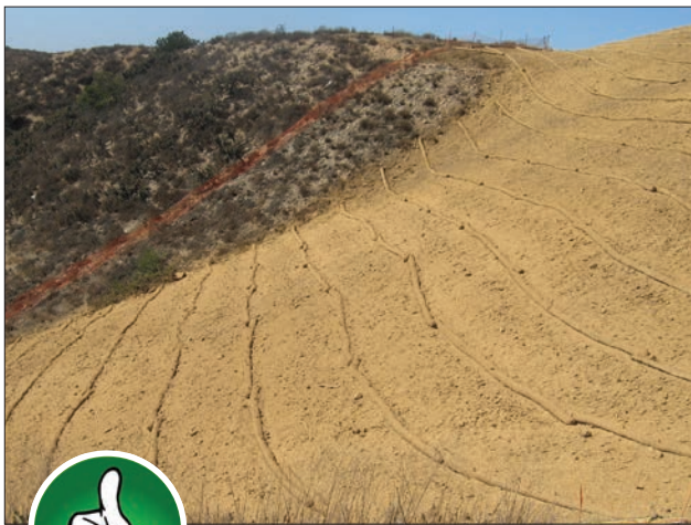
Fig. 1-1. Proper management of construction sites through the use of BMPs can dramatically reduce stormwater impacts. Source: RBF Consulting
