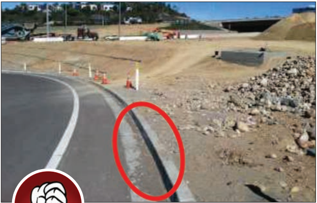
Fig. 3-3. Notice the sediment within the gutter caused by lack of perimeter controls.
