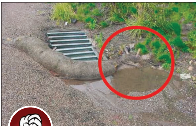
Fig. 5-15. Notice the stormwater that is bypassing the erosion log.
