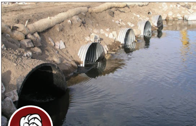
Fig. 5-5. Riprap with no fines should be installed at the approach to prevent sediment from entering the stream. If temporary, a silt fence could be used with sand bags anchoring the fabric on the culverts.
