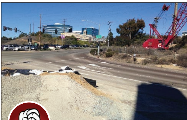
Fig. 3-15. Persistent sediment tracking may require street sweeping or a tire wash in combination with an entrance control (in this case, shaker plates).
