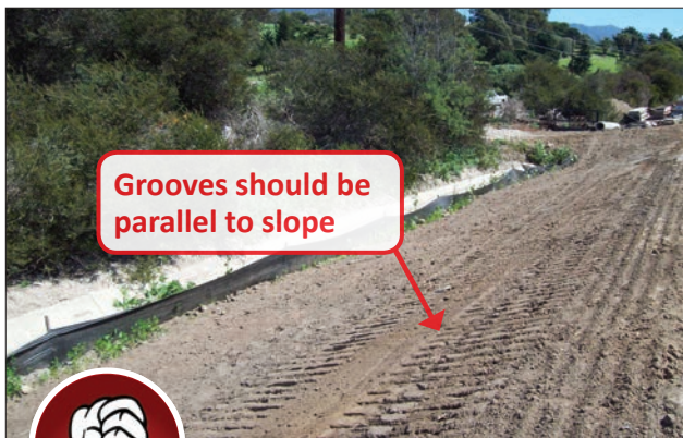
Fig. 4-3. Surface roughening is shown correct near the top of the slope; however shallow grooves in the lower half are in the wrong direction.
