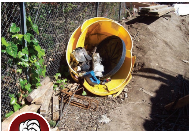
Fig. 2-12. Workers overlook placement of small amounts of waste material such as this in proper disposal areas.
